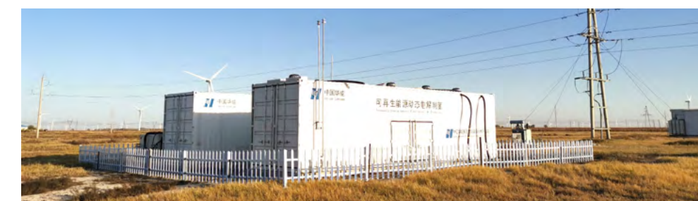
Wind Power Dynamic Electrolytic Hydrogen Production Demonstration Project
