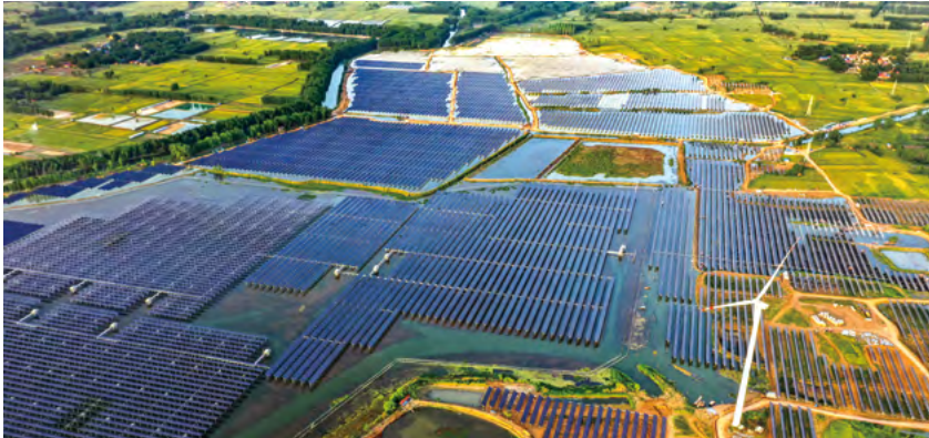
Huaiyin Power Plant's Sihong 100MW PV Pioneer Power Generation Project
