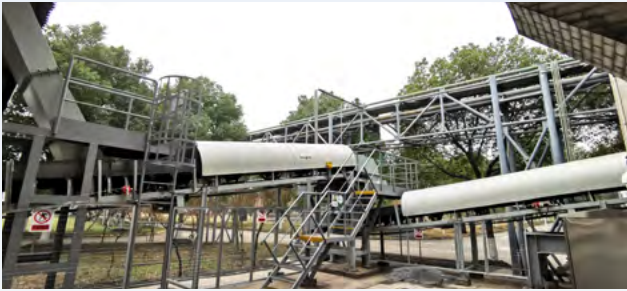
Sludge Power Generation Project of Suzhou Thermal Power Plant
