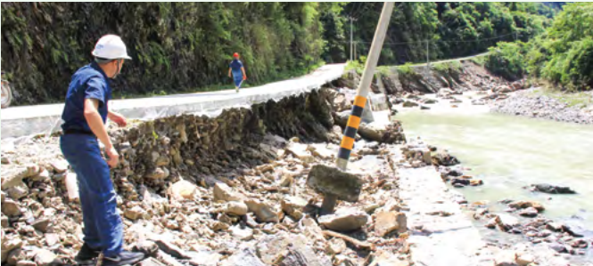
Entrance Road to the Dam Qinglong Hydropower Station was Damaged
