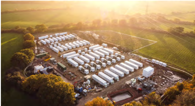
China Huaneng UK Minety Battery Storage Project
