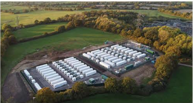
China Huaneng UK Minety Battery Storage Project
